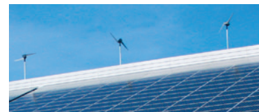
Schedetal Energiedach Sonne | Wind
